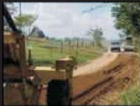
Installation in Panama with Cat 250r stabilizer machine then sealed with LDC
